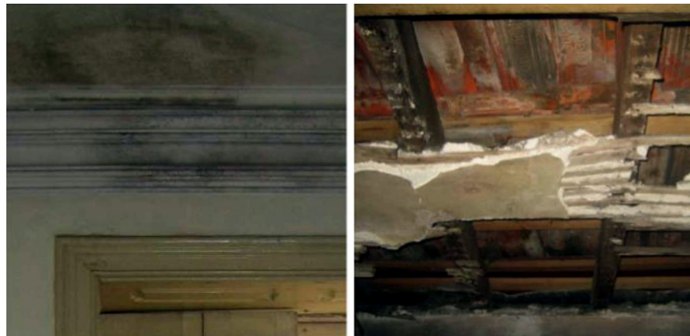
a) Mold stains
