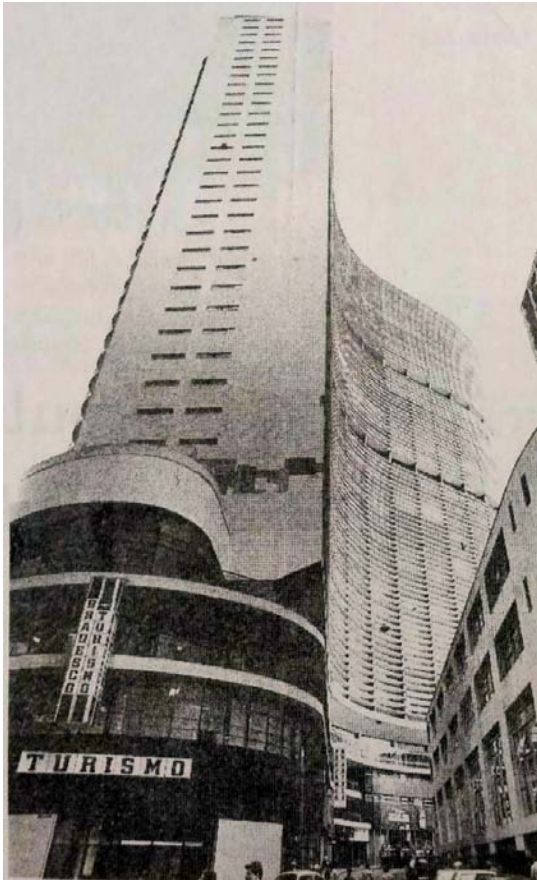
Figure 6 – Degradation of the façade published in 1991 by the newspaper Folha de S.Paulo Source: Copan Archive.
